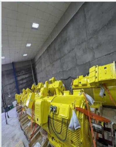
Mill Main Motor Indoor storage
