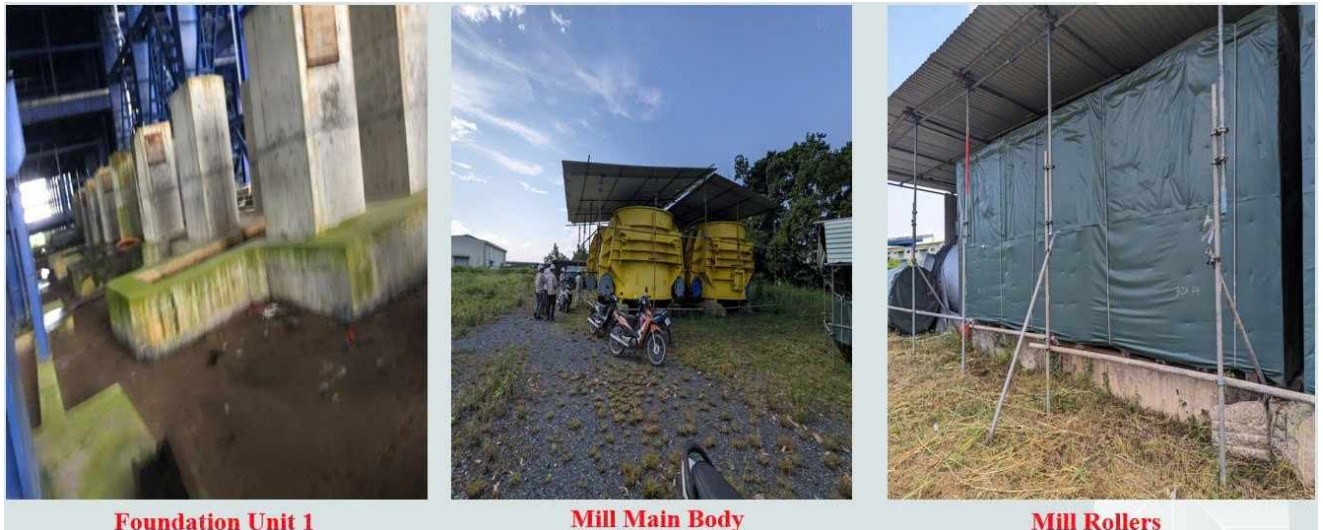
Photo: Coal Mills at Site
