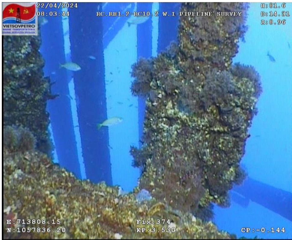
Figure 17: Riser clamp at EL -15m
