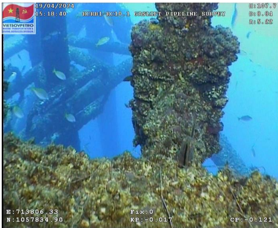
Figure 5: Riser clamp at EL -10m
