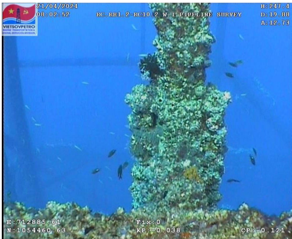
Figure 7: Riser clamp at EL -21m
