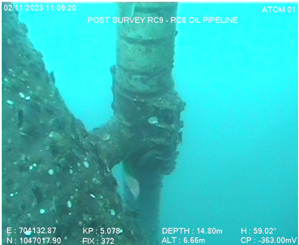
Figure 8: Riser clamp at EL: -14m
