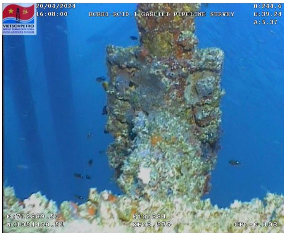
Figure 23: Riser clamp at EL -40m
