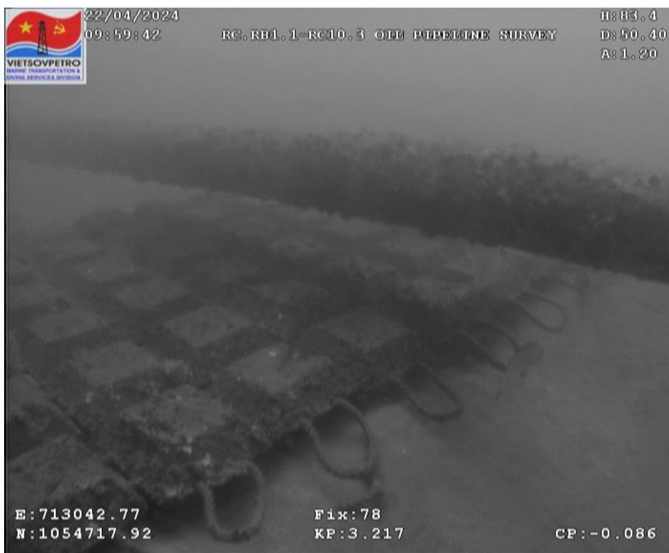
Figure 49: Concrete mattress #9 not supporting
