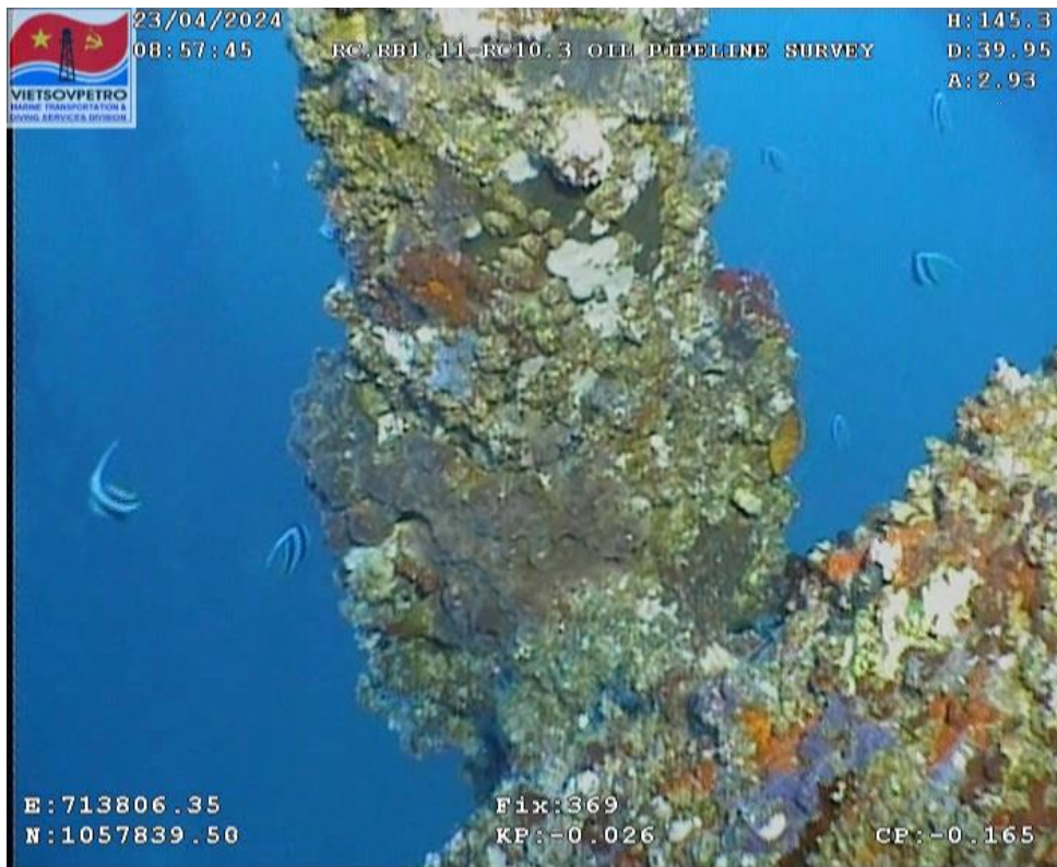
Figure 20: Riser clamp at EL -41m
