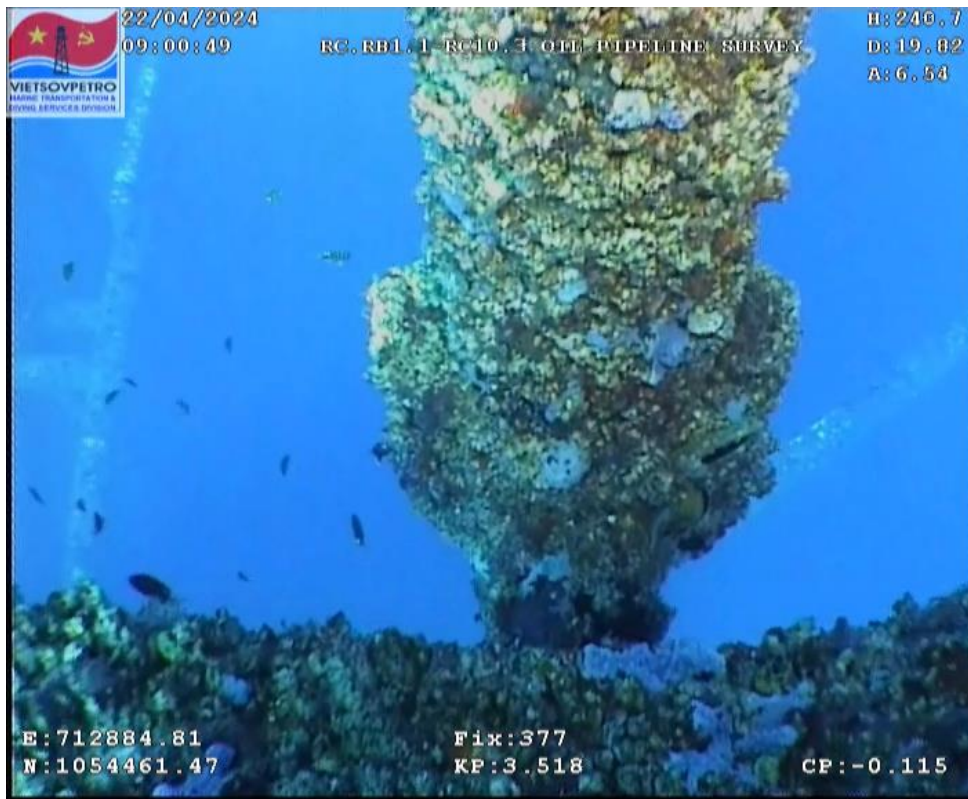
Figure 6: Riser clamp at EL -21m
