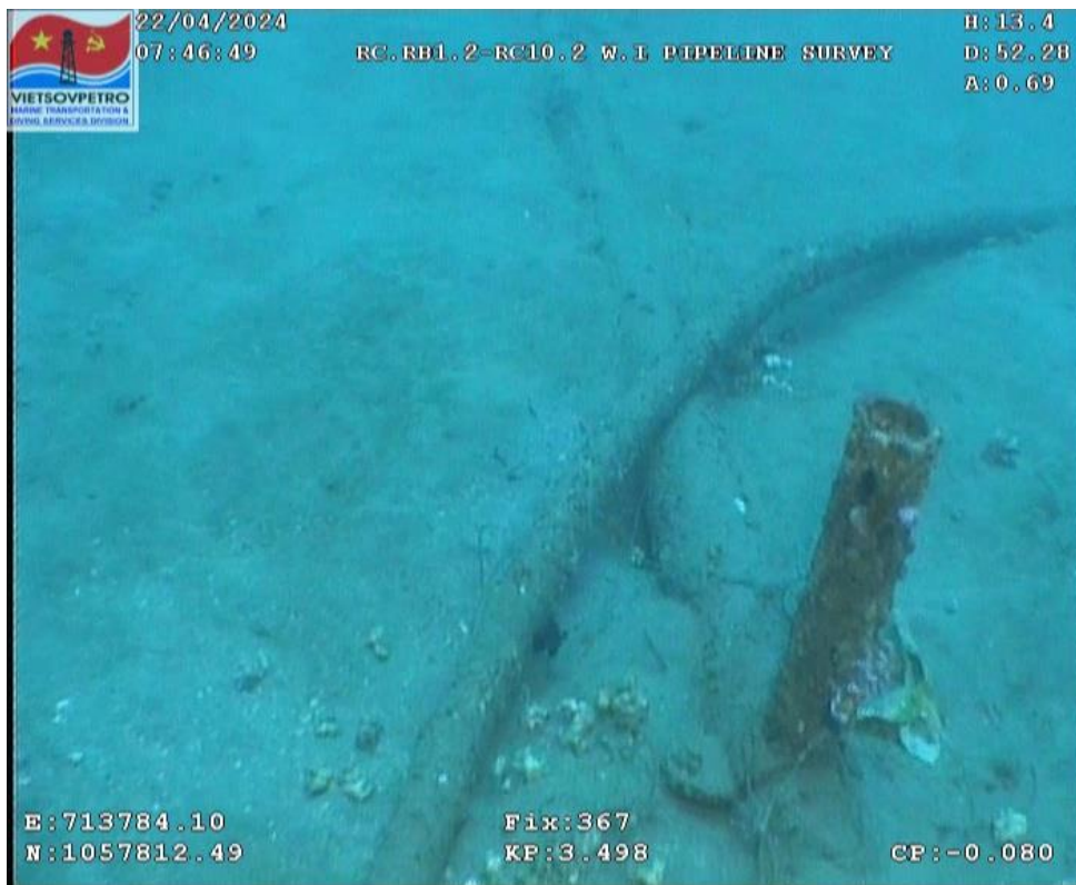
Figure 30: Crossing under power cable without support at Fix.367
