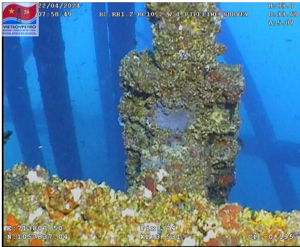
Figure 21: Riser clamp at EL -34m
