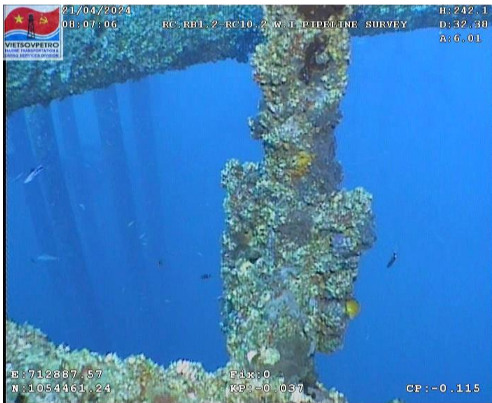
Figure 9: Riser clamp at EL -34m
