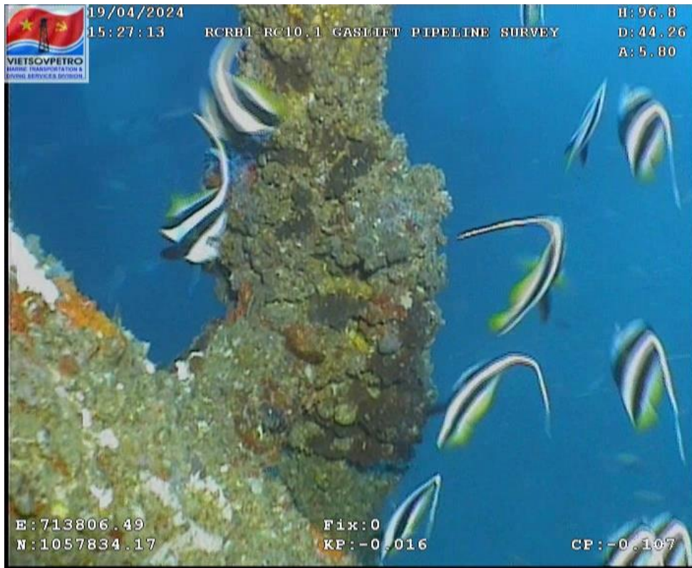
Figure 12: Riser clamp at EL -46m
