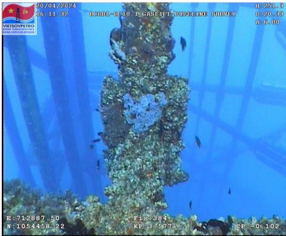
Figure 20: Riser clamp at EL -21m
