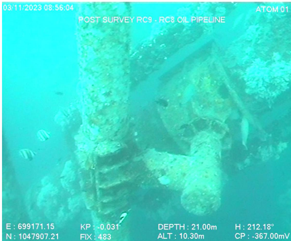
Figure 15: Riser clamp at EL: -21m
