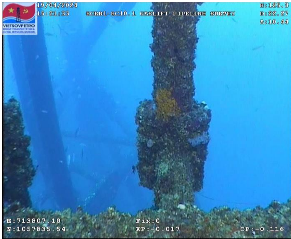
Figure 8: Riser clamp at EL -24m
