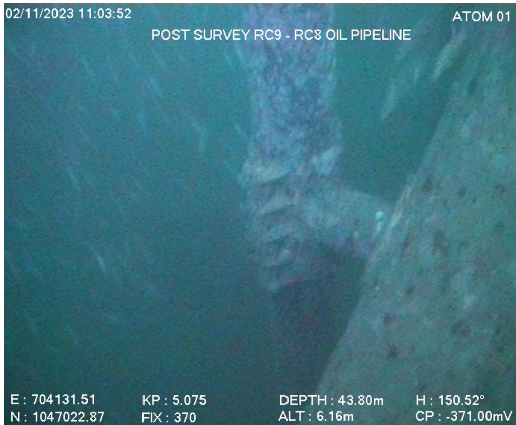
Figure 3: Riser clamp at EL: -46m
