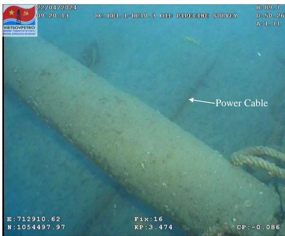
Figure 25: Crossing over power cable at Fix.16
