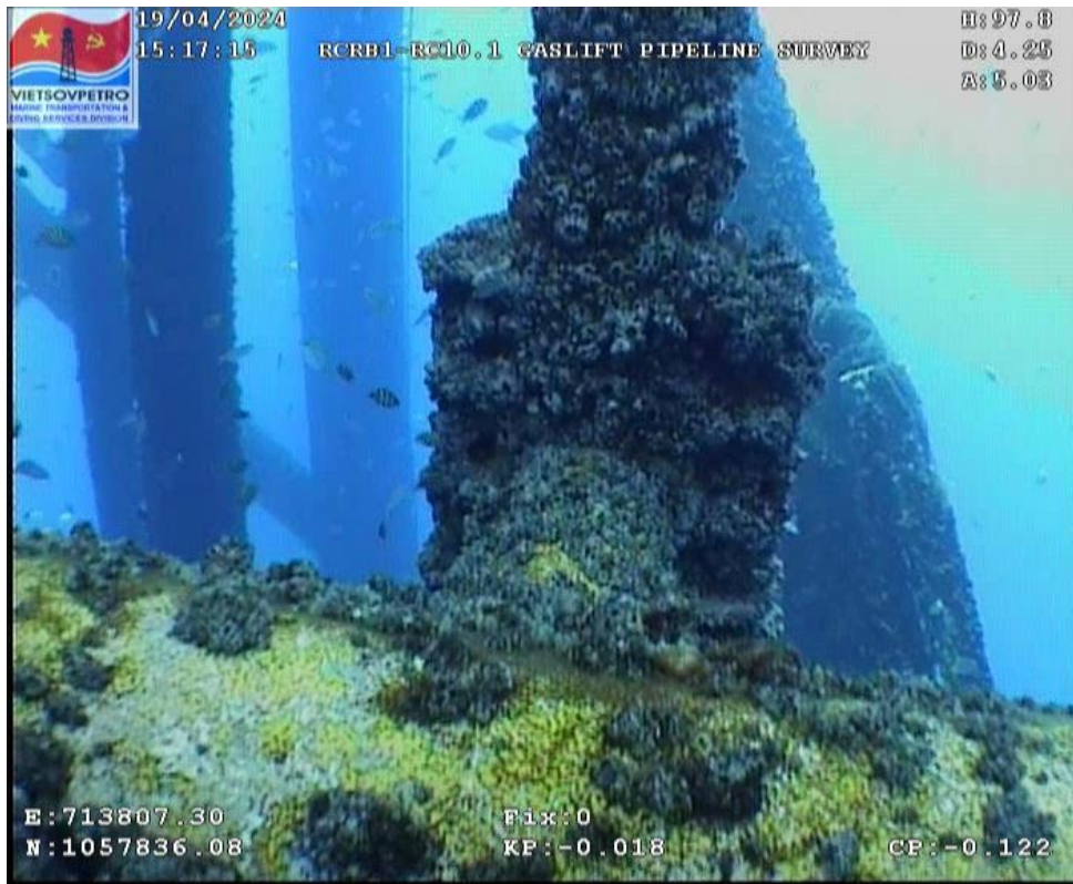
Figure 4: Riser clamp at EL -5m
