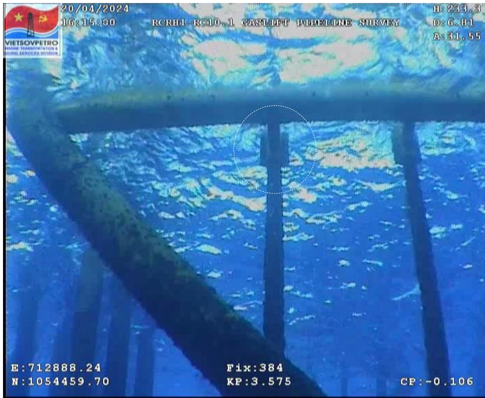
Figure 16: Riser clamp at EL -1m
