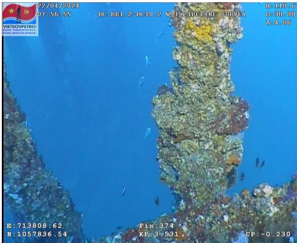
Figure 22: Riser clamp at EL -40m
