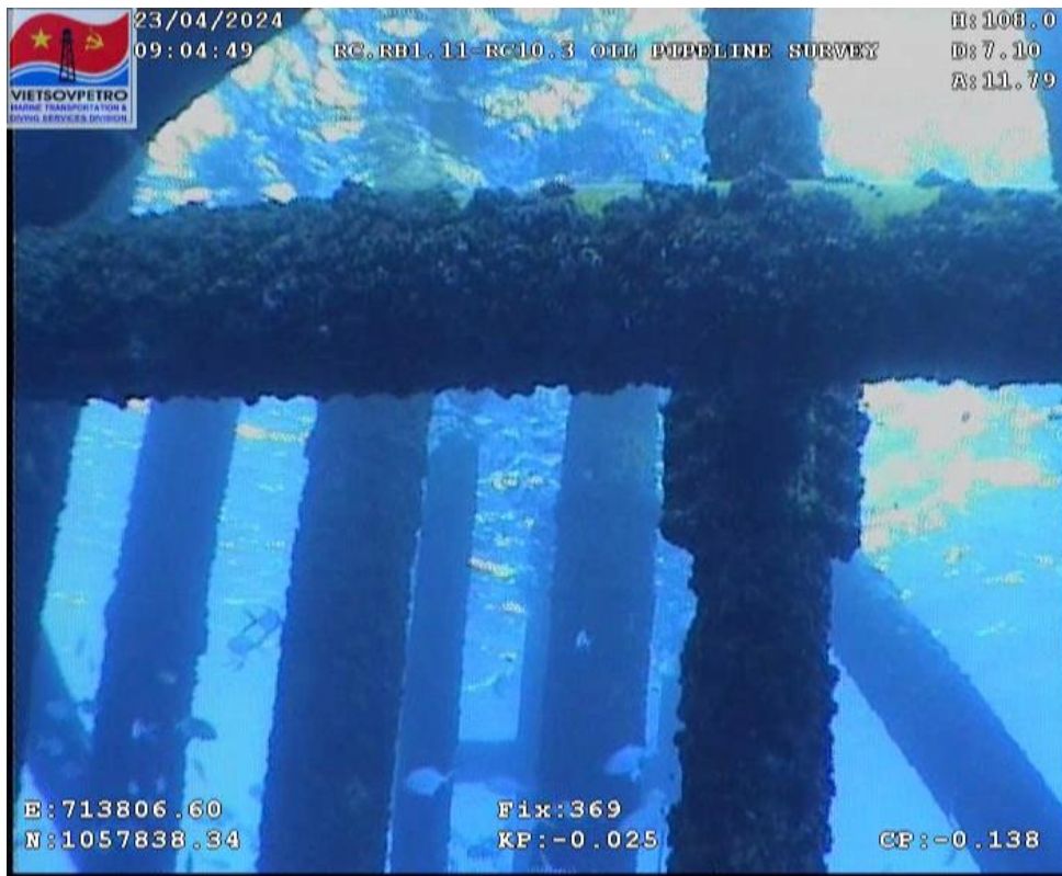
Figure 13: Riser clamp at EL -5m
