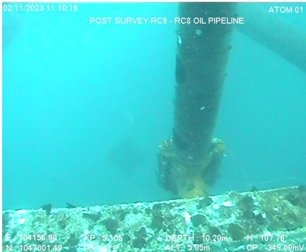
Figure 9: Riser clamp at EL: -11m
