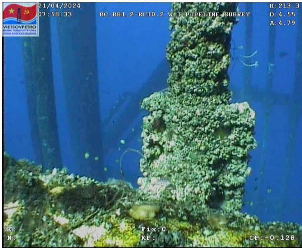
Figure 4: Riser clamp at EL -5m
