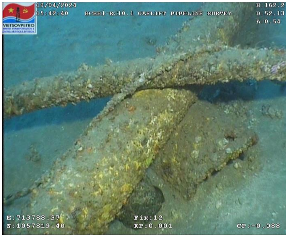
Figure 28: Crossing under power cable without support at Fix.12
