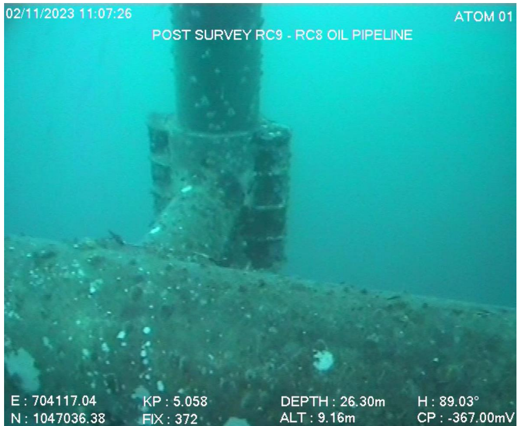
Figure 6: Riser clamp at EL: -27m
