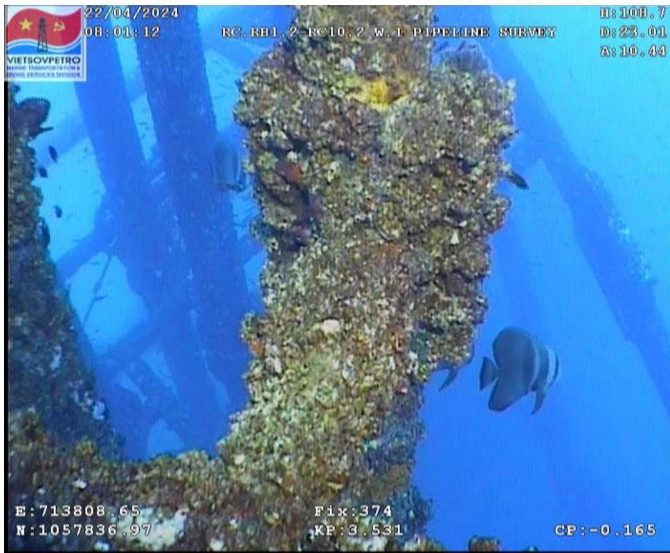
Figure 19: Riser clamp at EL -24m
