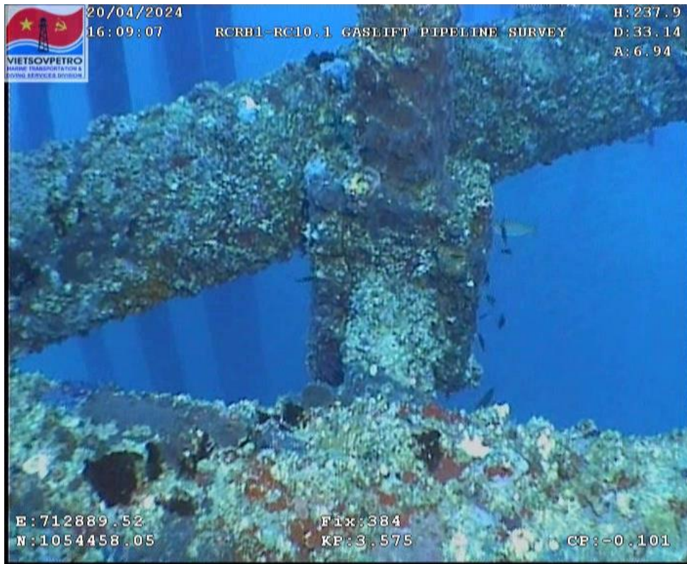
Figure 22: Riser clamp at EL -34m
