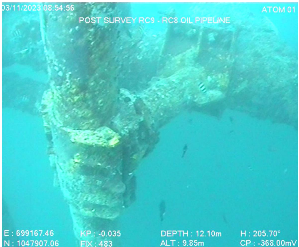
Figure 14: Riser clamp at EL: -12m
