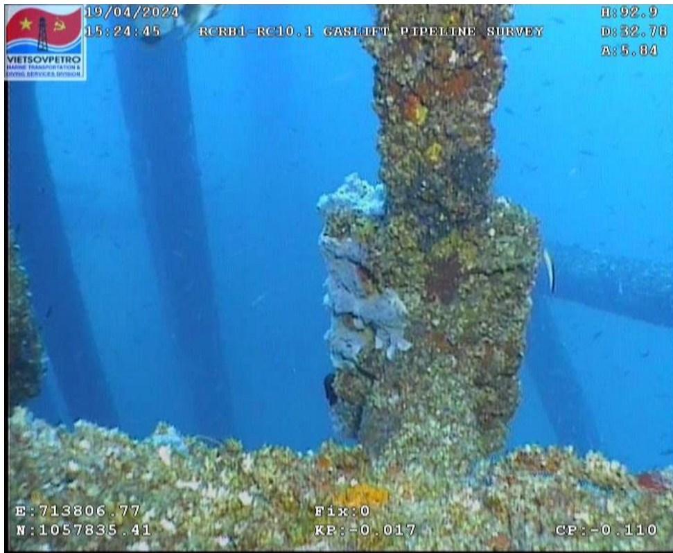
Figure 10: Riser clamp at EL -35m
