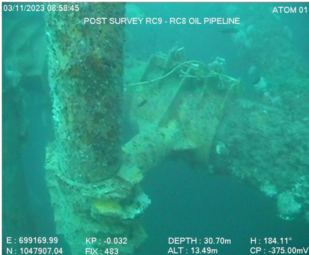
Figure 16: Riser clamp at EL: -30m
