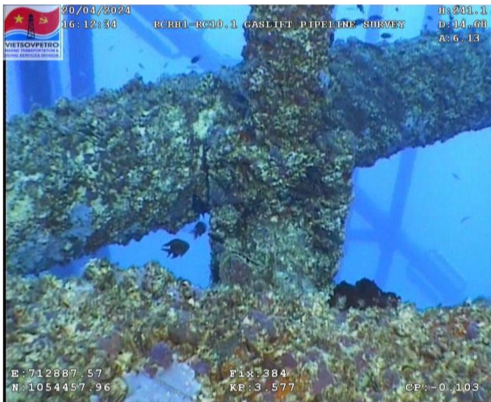
Figure 19: Riser clamp at EL -15m
