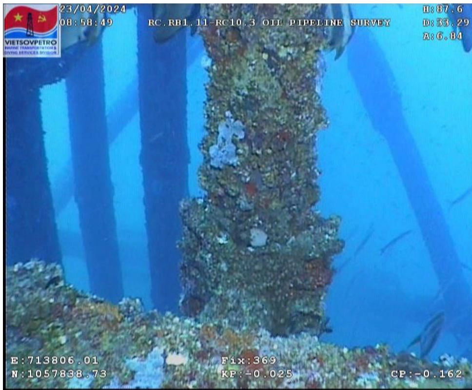
Figure 19: Riser clamp at EL -35m
