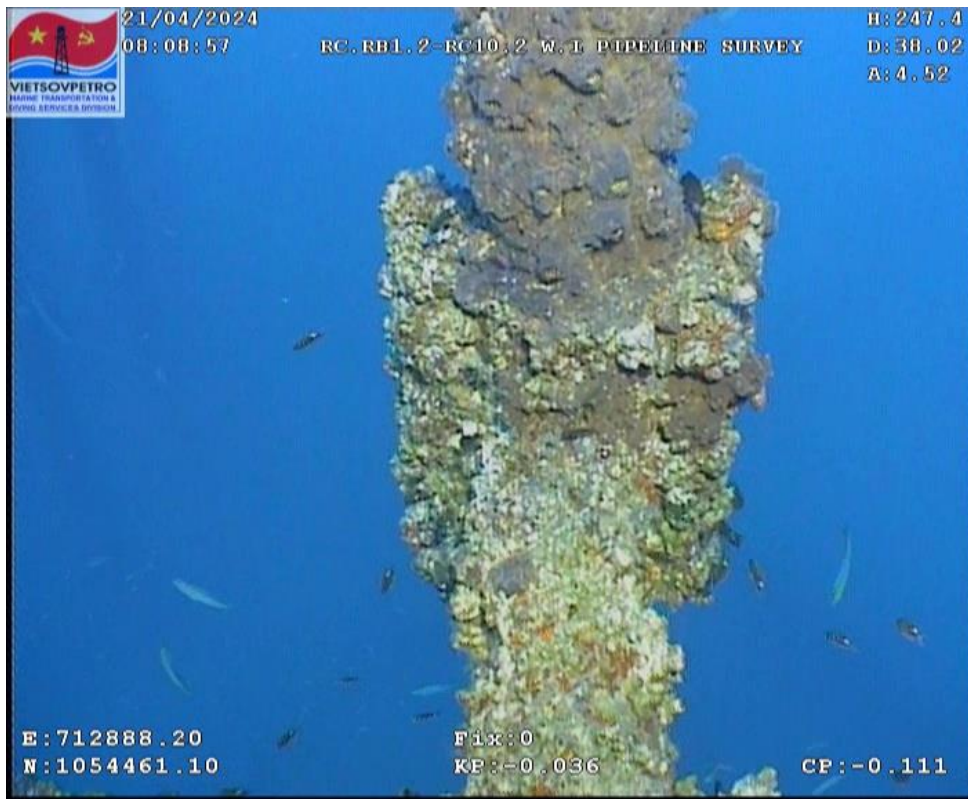
Figure 10: Riser clamp at EL -39m
