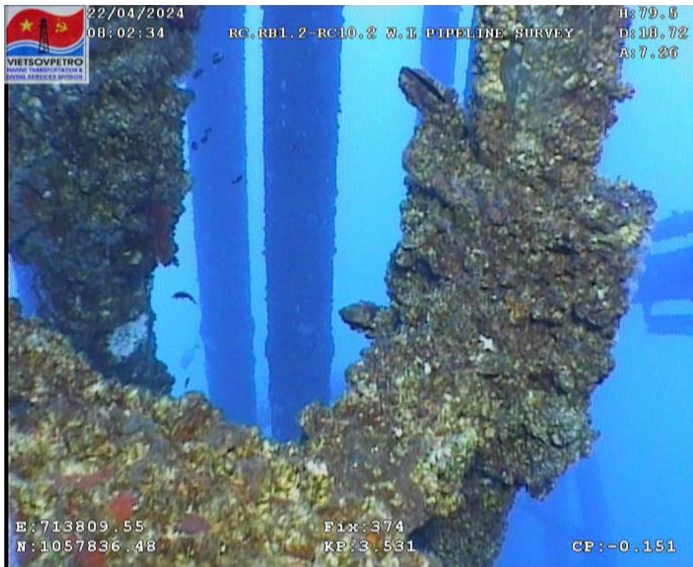
Figure 18: Riser clamp at EL -20m
