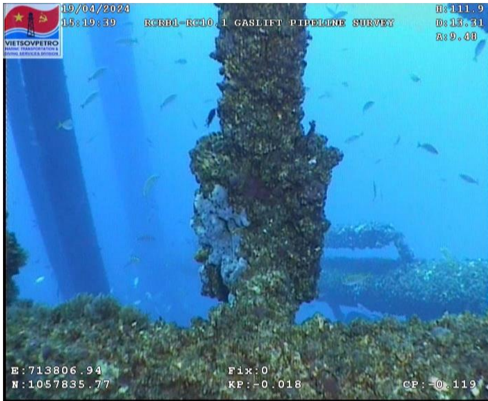
Figure 6: Riser clamp at EL -15m
