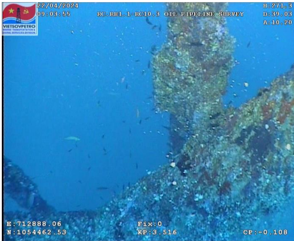
Figure 9: Riser clamp at EL -41m
