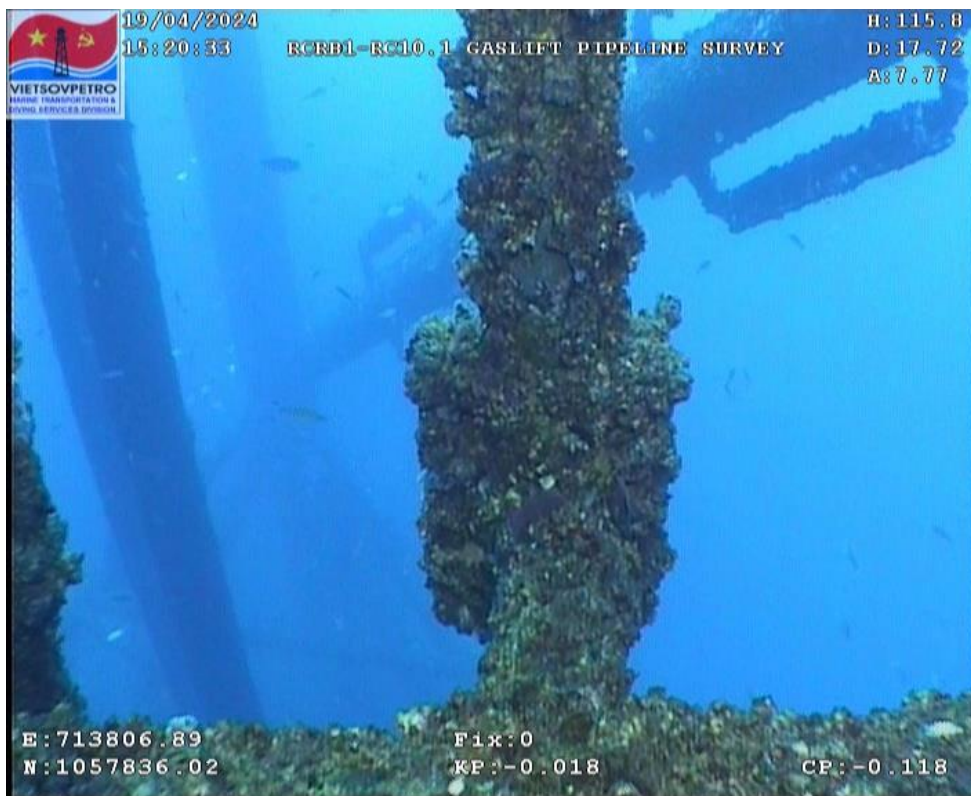
Figure 7: Riser clamp at EL -20m
