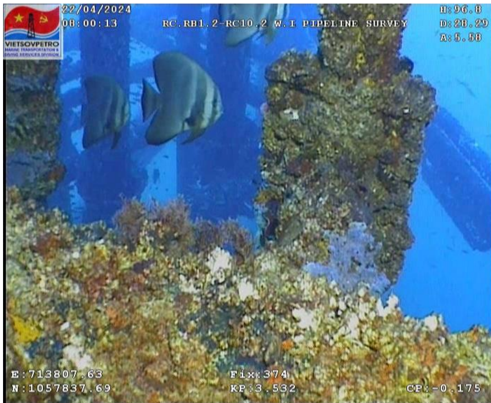
Figure 20: Riser clamp at EL -29m
