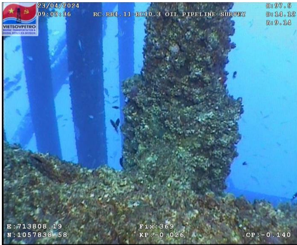
Figure 15: Riser clamp at EL -15m
