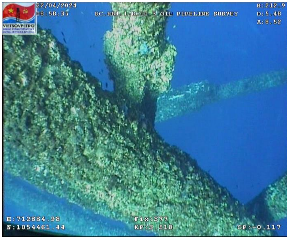
Figure 4: Riser clamp at EL -7m
