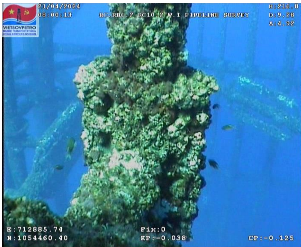
Figure 5: Riser clamp at EL -10m
