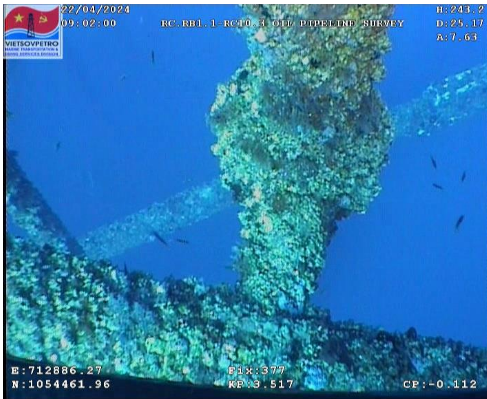
Figure 7: Riser clamp at EL -26m
