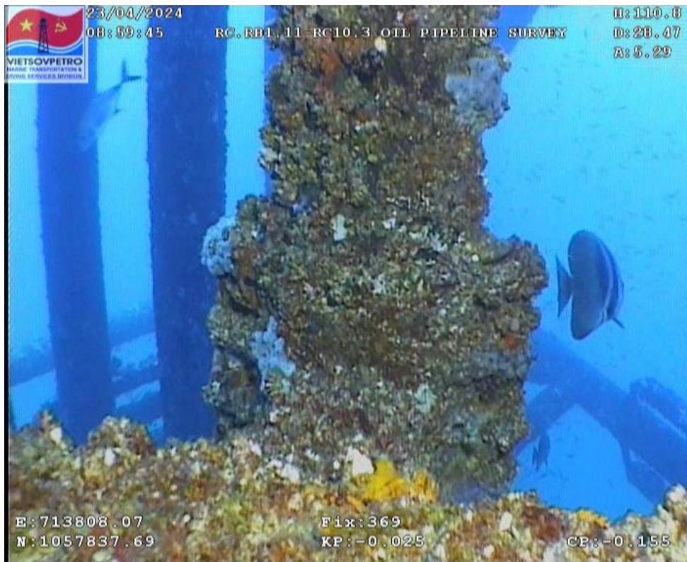
Figure 18: Riser clamp at EL -29m
