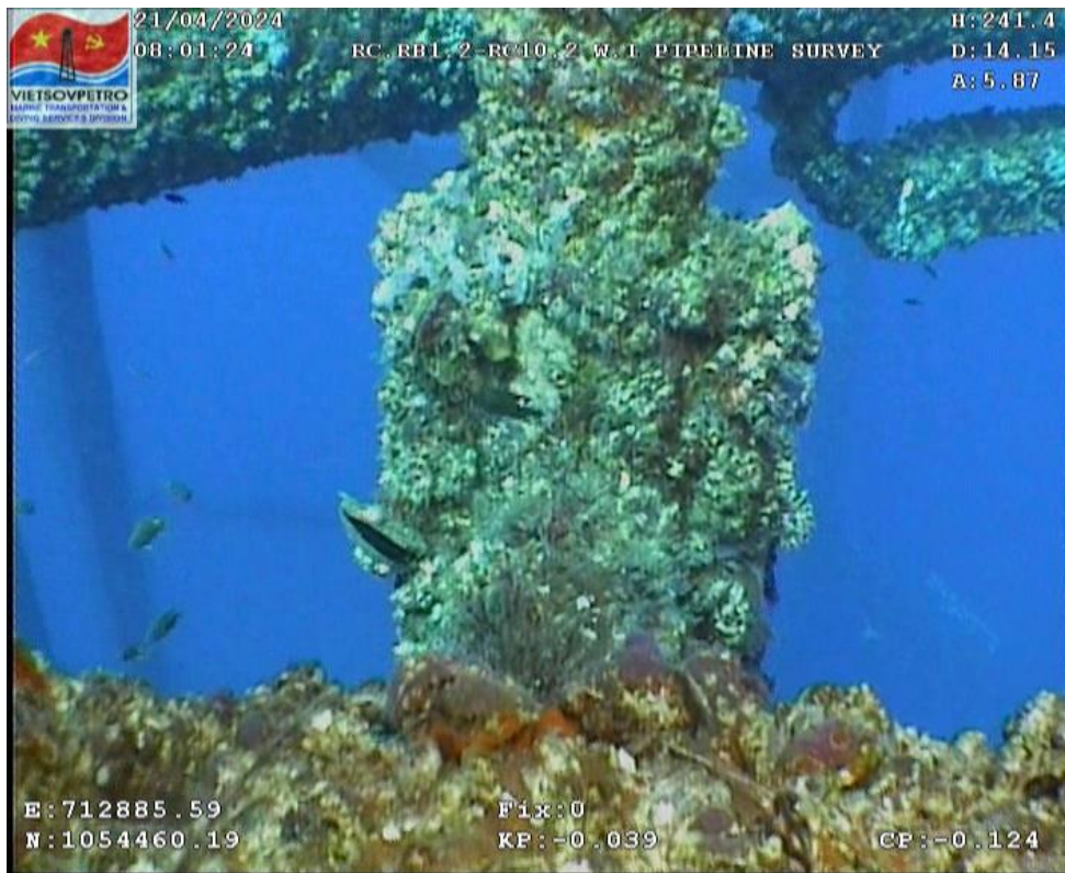
Figure 6: Riser clamp at EL -15m
