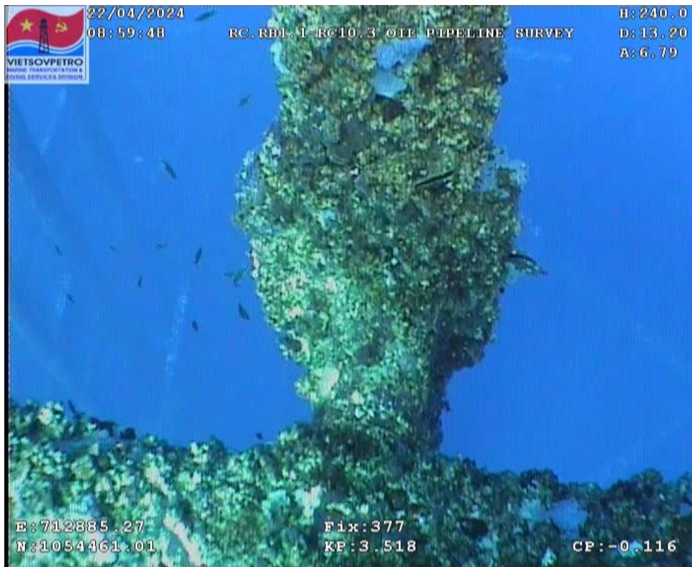
Figure 5: Riser clamp at EL -14m
