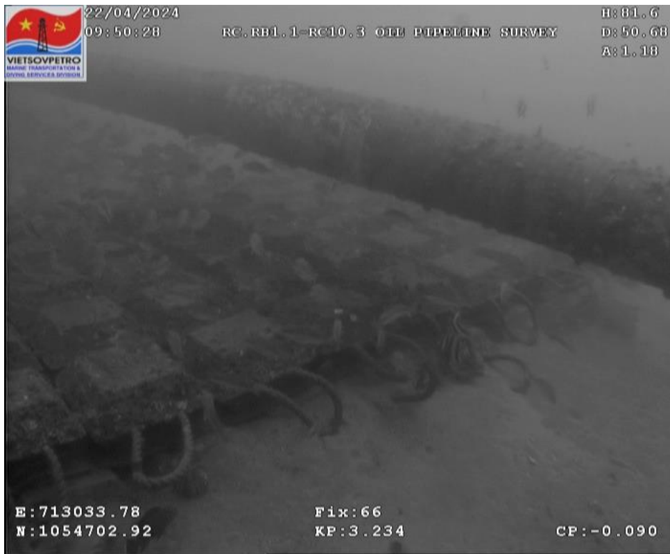
Figure 47: Concrete mattress #7 not supporting
