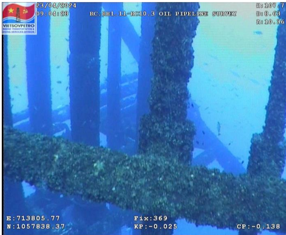
Figure 14: Riser clamp at EL -10m
