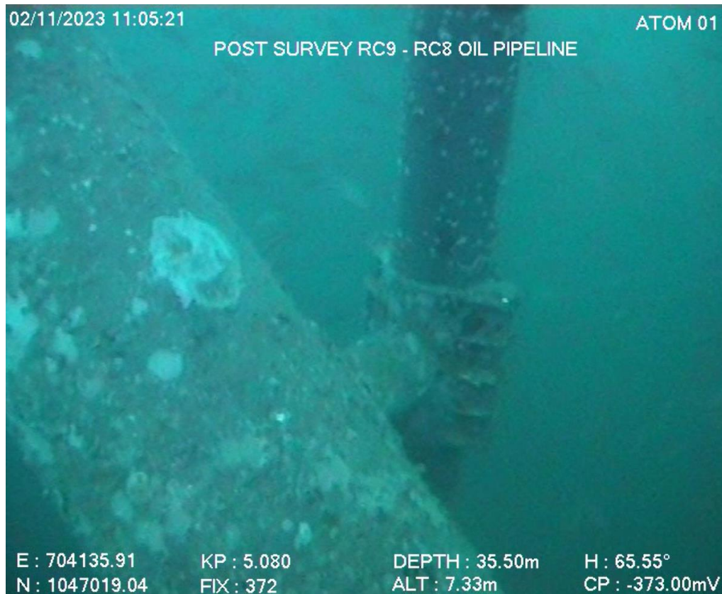
Figure 4: Riser clamp at EL: -38m
