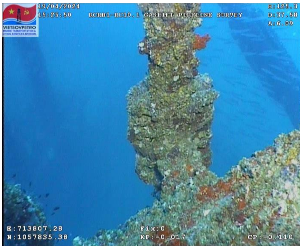
Figure 11: Riser clamp at EL -39m
