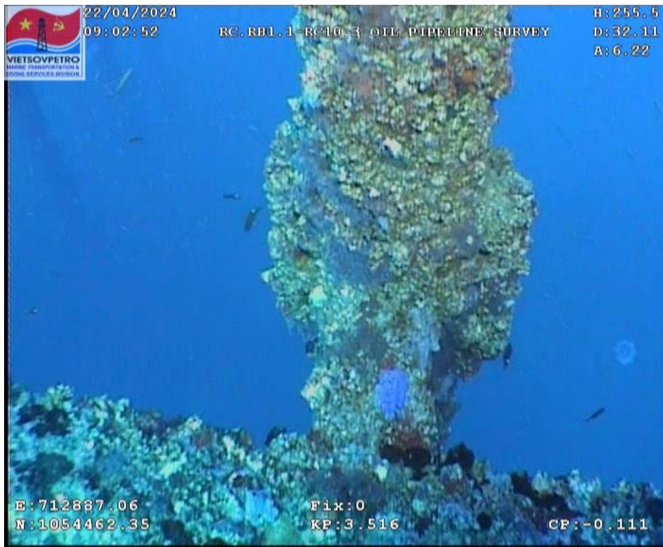
Figure 8: Riser clamp at EL -33m
