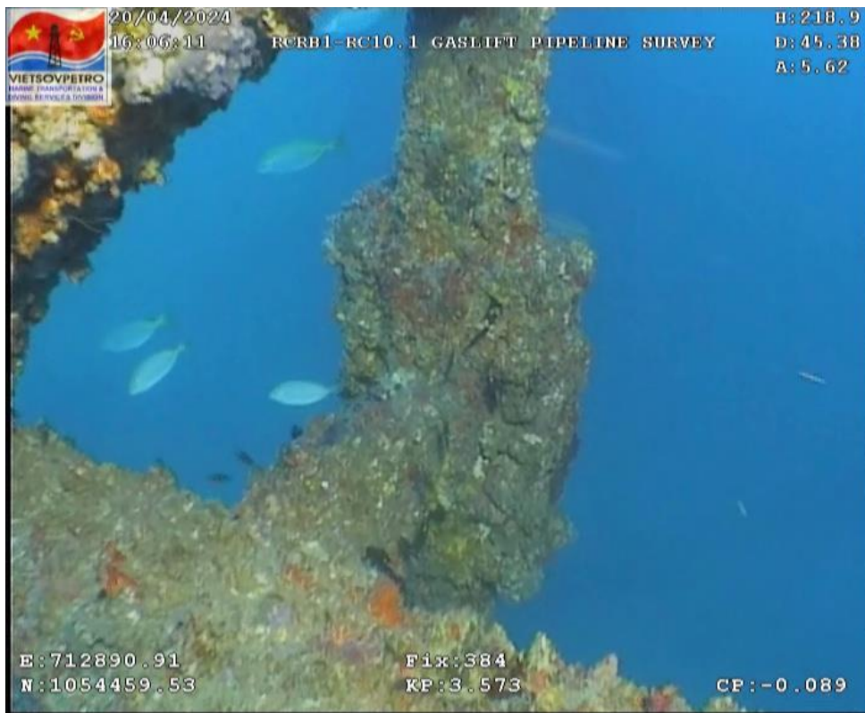
Figure 24: Riser clamp at EL -46m
