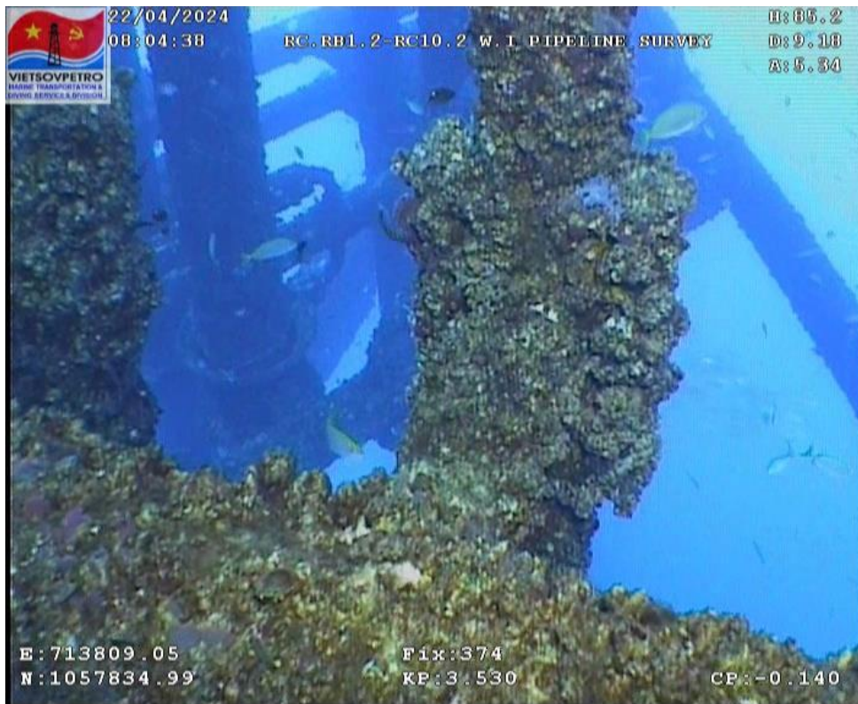
Figure 16: Riser clamp at EL -10m
