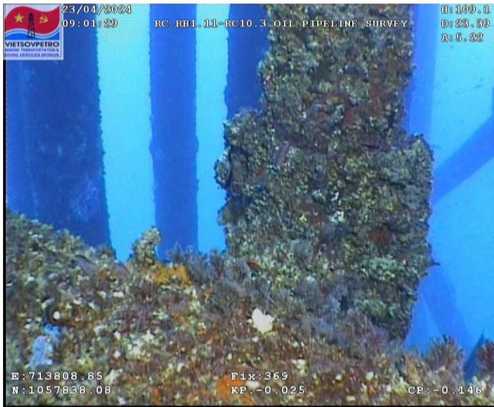
Figure 17: Riser clamp at EL -24m
