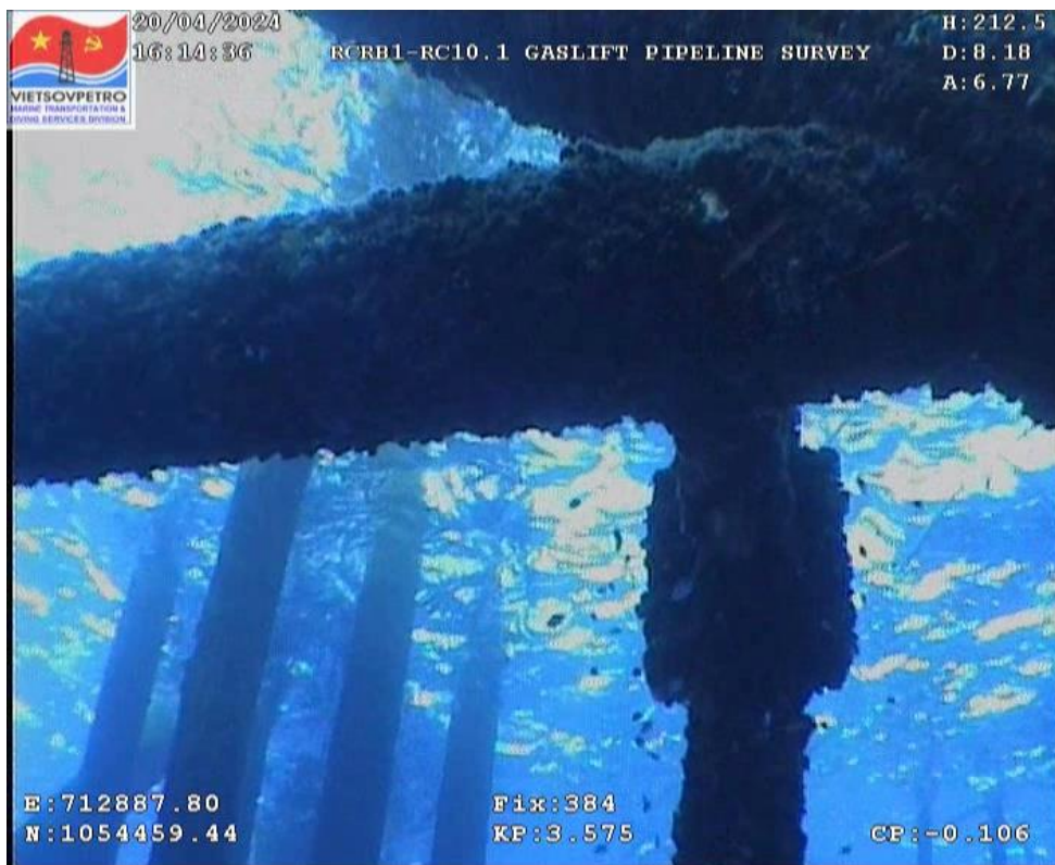
Figure 17: Riser clamp at EL -6m
