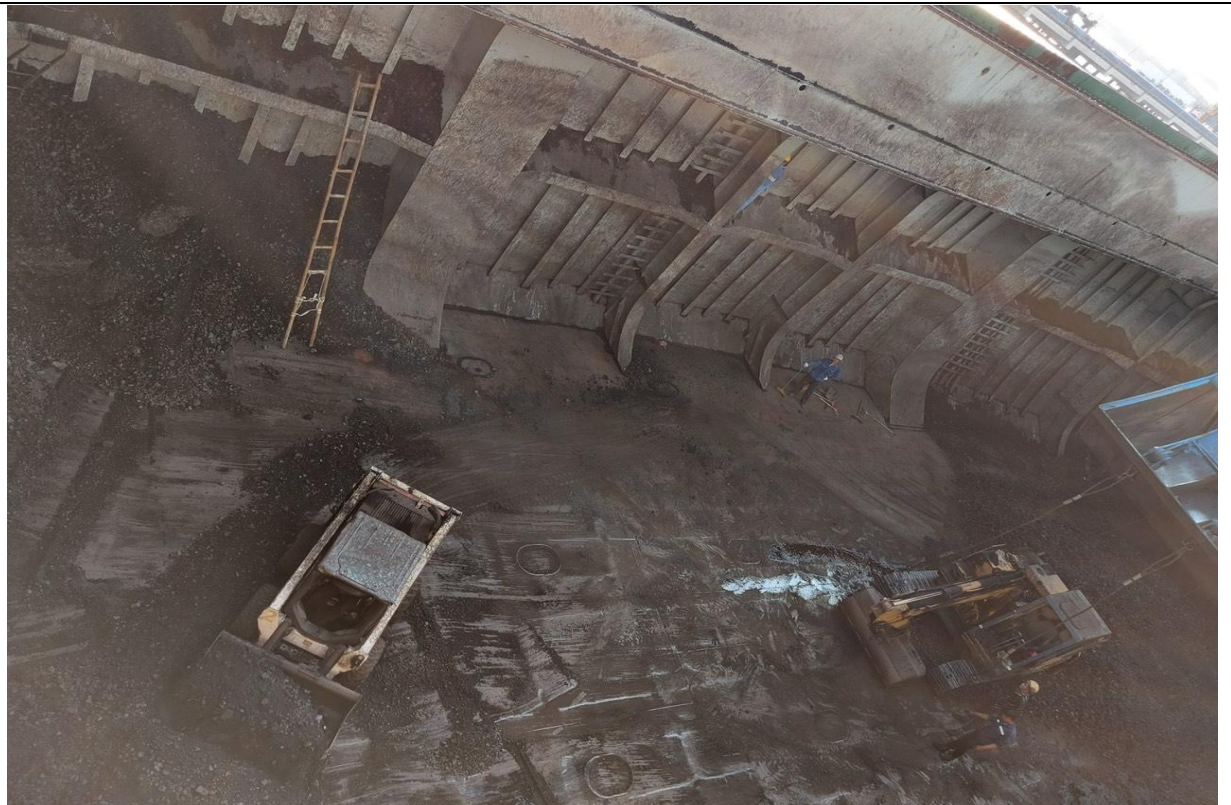
Vessel/berth with vertical keel being exposed and extended to the bottom of the cargo hold, horizontal keel being exposed and dragged along the cargo hold. The bottom of the cargo hold is flat
