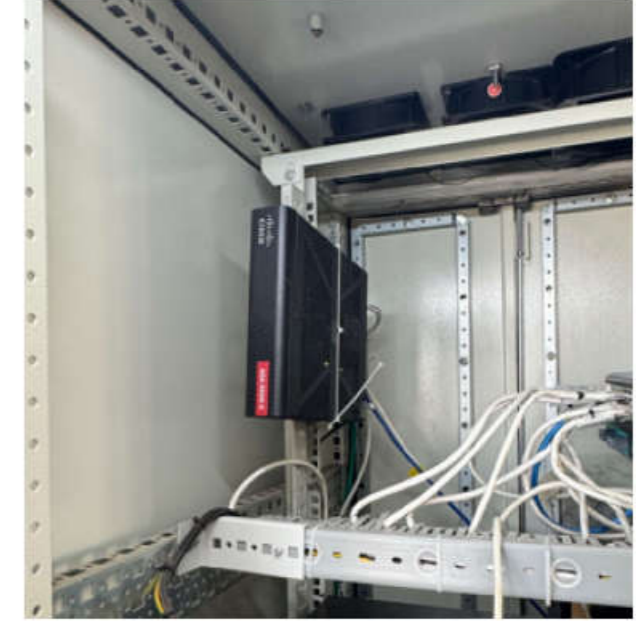
FIREWALL SẼ THU HỒI TBA 110KV MANG YANG
