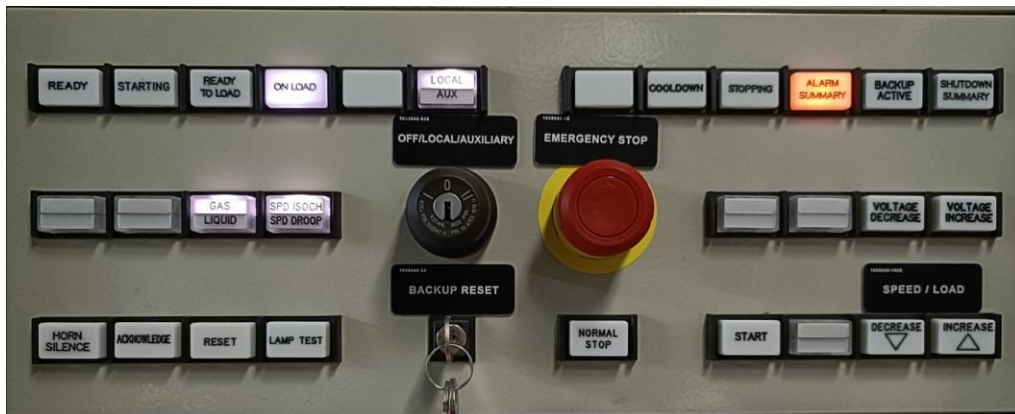
Turbine Control Panel
